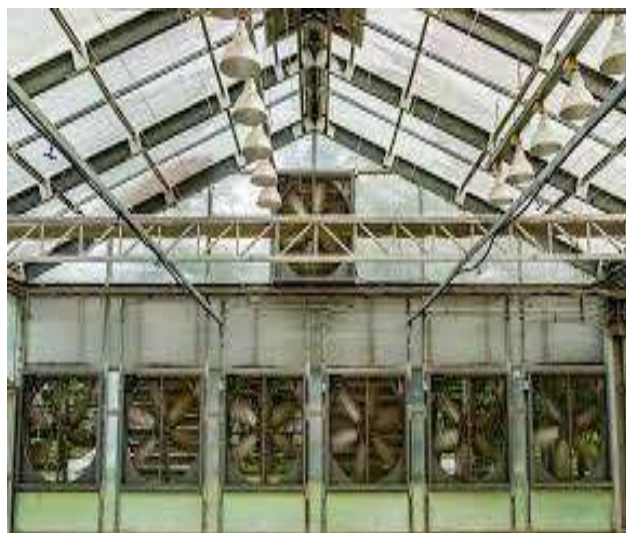
Figure No 125 Greenhouse for active heating
