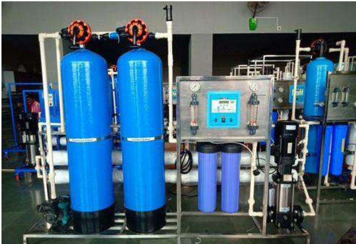
Figure No 91. R.O. Water Plant
