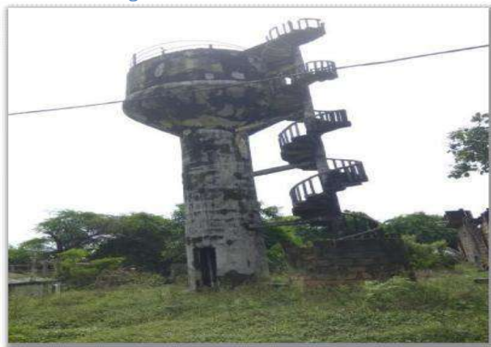
Figure No 47. Over head Tank
